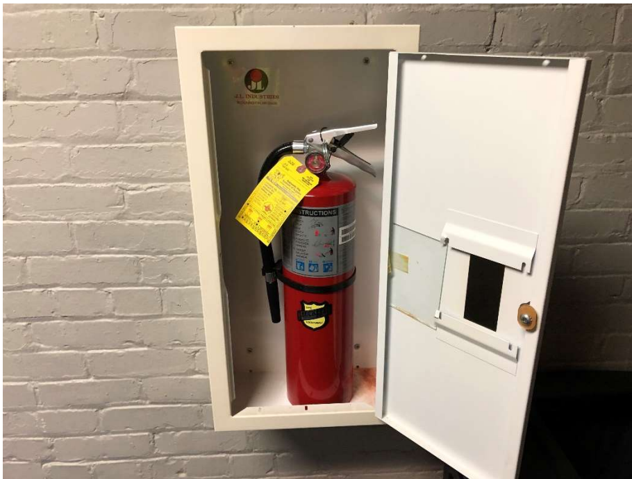
Photograph 10: Typical view of a fire extinguisher located at the Subject Property.
