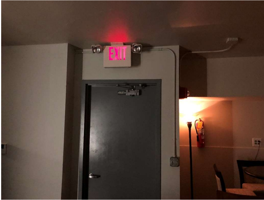
Photograph 7: Typical view of an exit sign located at the Subject Property.
