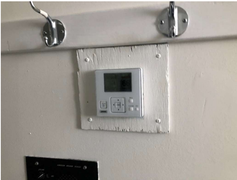
Photograph 6: Typical view of an electronic thermostat located at the Subject Property.
