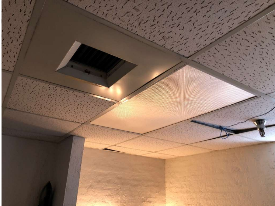
Photograph 1: Typical view of the 4' Fluorescent light ballasts located at the Subject Property.
